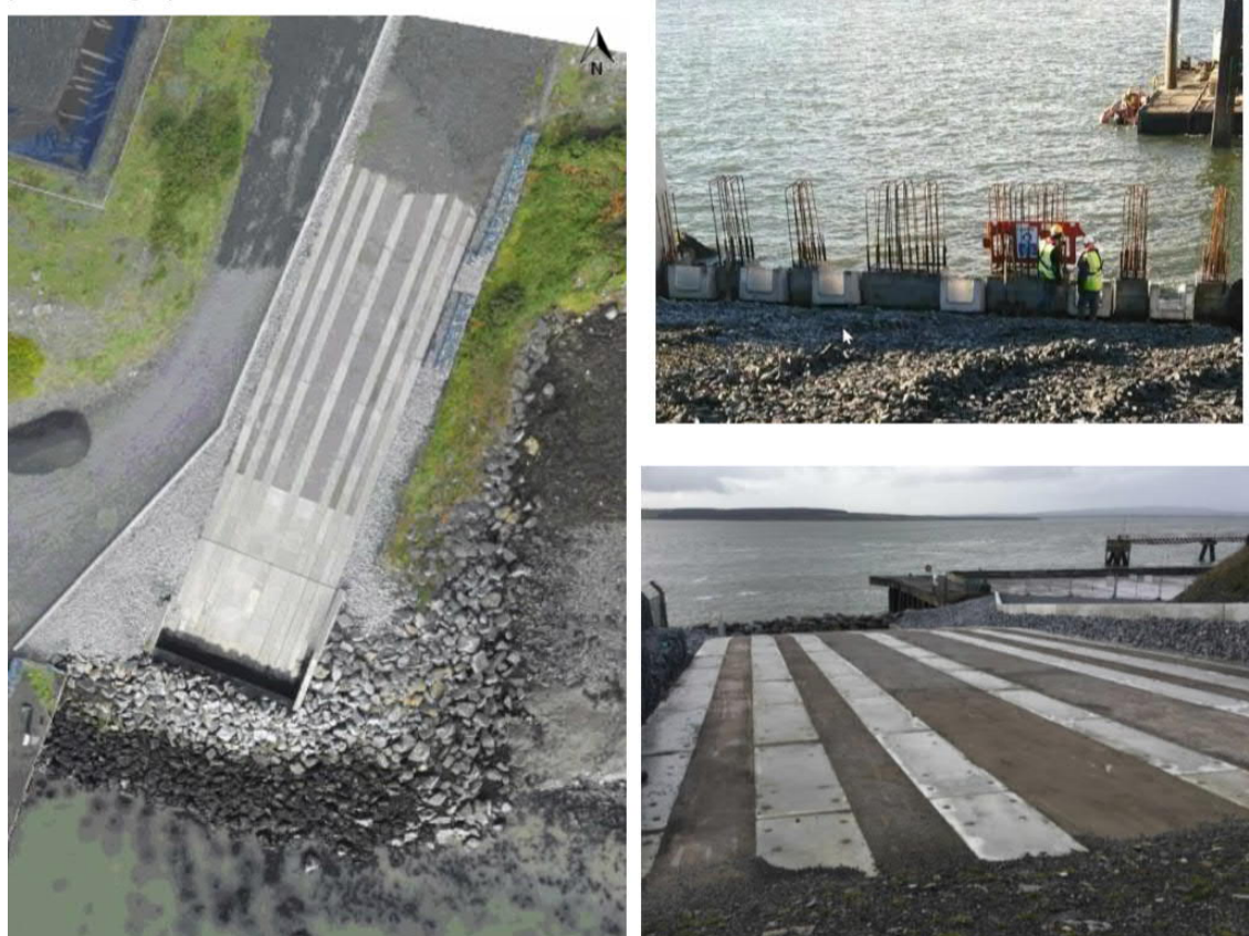
Figure 2.27: Concrete 'slipway' structure at Moneypoint. A similar landfall design is proposed for the 400 kV cable landfall works. Aerial view (left), cable trough installation (top right) and top surface (bottom right Kilpaddoge Landfall Works (Step 1b))
